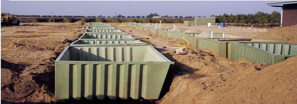
Irrigation distribution system already installed on 2.6 acres of open ground. Trees have been removed. Designed for 16 reps.
